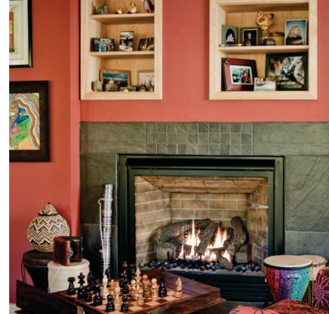
This gas fire helps to warm the room, along with an air handler attached to the upper portion of the wall. The air handler is part of a ductless Sanyo minisplit system. The house has six air handlers, three upstairs and three downstairs.
